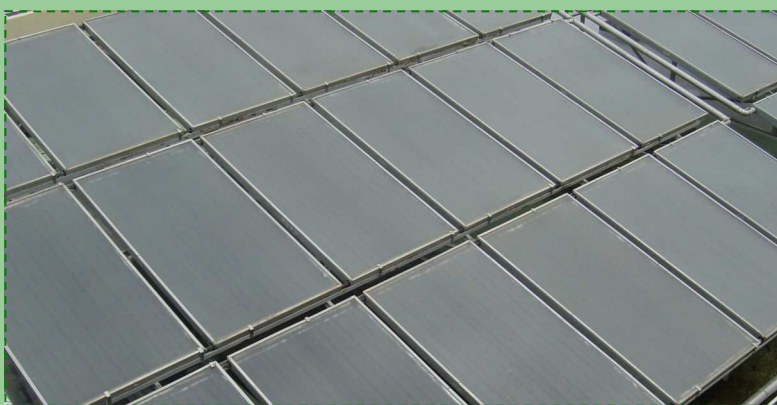
Solar Thermal Plant for Hot water
